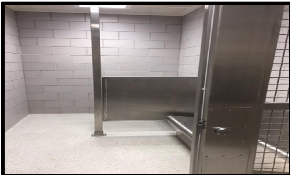
USMS prisoner holding cell constructed to current standards.
