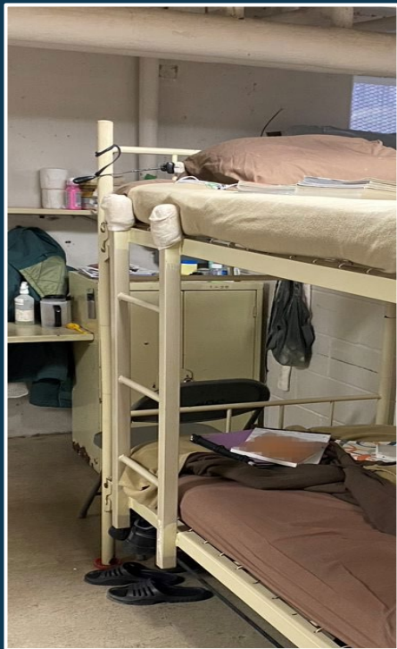
Proximity of exposed pipes to inmate beds in FCI Waseca
