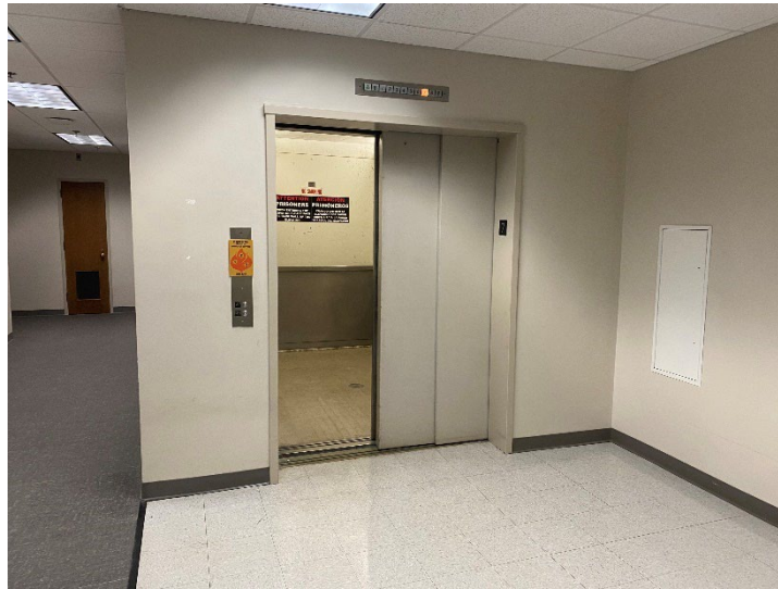
Raleigh, NC – Existing freight elevator used for prisoner movement will be replaced by a new prisoner elevator by a current Capital Security Program project.
