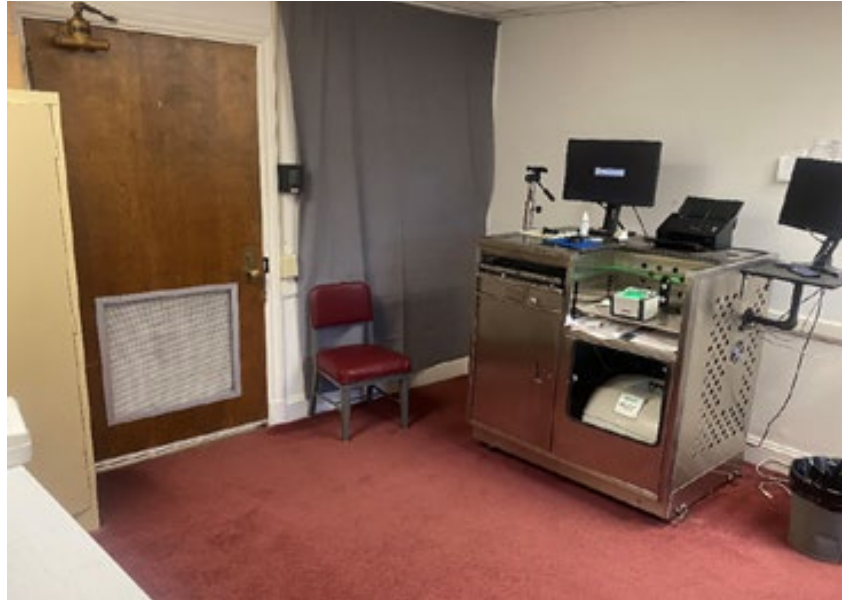
Location withheld – Prisoner processing room (carpeting drywall, unsecure door). Secure lock on door, but kickout vent leads to unsecure area.
