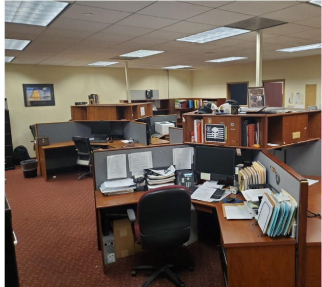
Camden, NJ – Worn carpet with trip hazards; outdated, deteriorating furniture needs to be replaced with more space efficient systems furniture.
