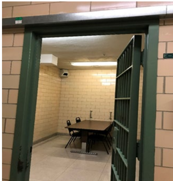
Washington, DC – District Court interview room. No prisoner/attorney separation, plaster ceilings, antiquated door does not provide sight/sound separation.
