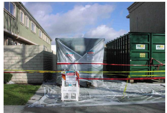
Defendant Yi Disposed of Asbestos in this Solid Waste Dumpster.
