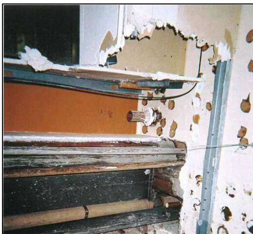
Exposed Asbestos in the Wall of the Equitable Building Iowa Department of Natural Resources Photo
